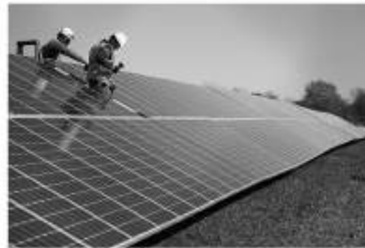
Designing of photovoltaic plants with output of 600 MW, 150 MW realized
